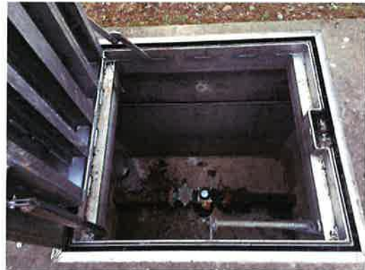
Source Meter Vault
