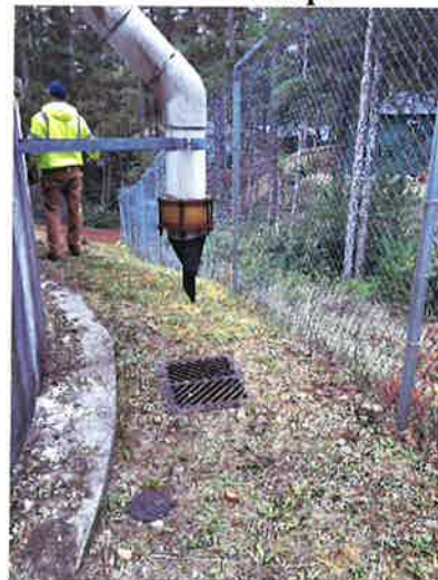
Overflow Air Gap
