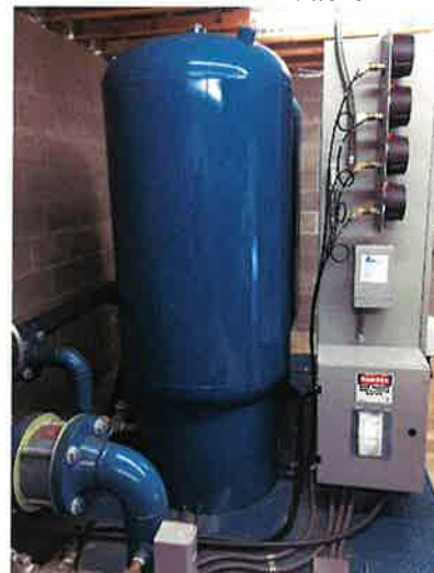
Booster Station Skid
