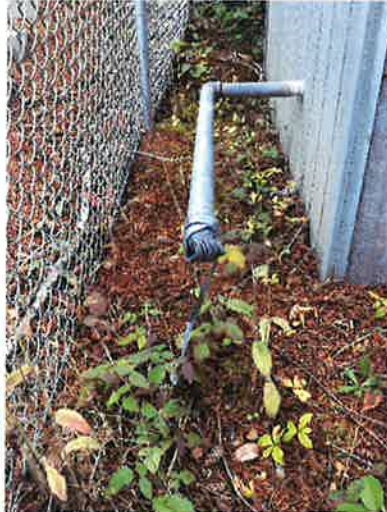
Discharge Line from Booster Station
