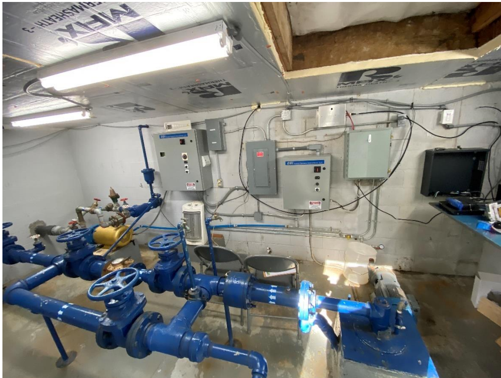
Figure 4: Well 4 Electrical Equipment
