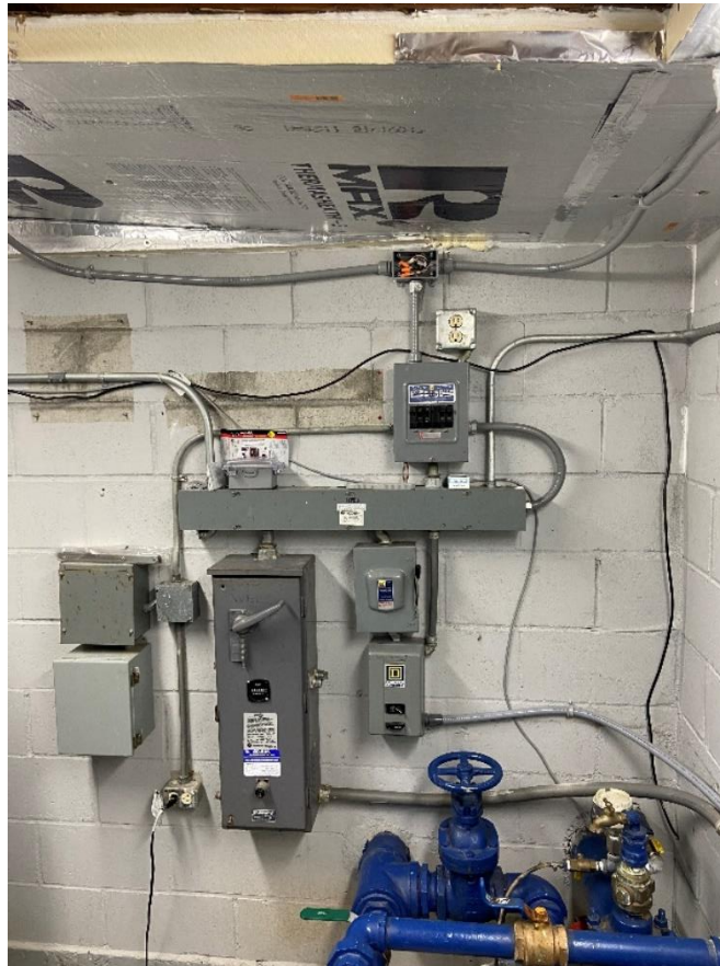
Figure 1: Well 1 Electrical Equipment
