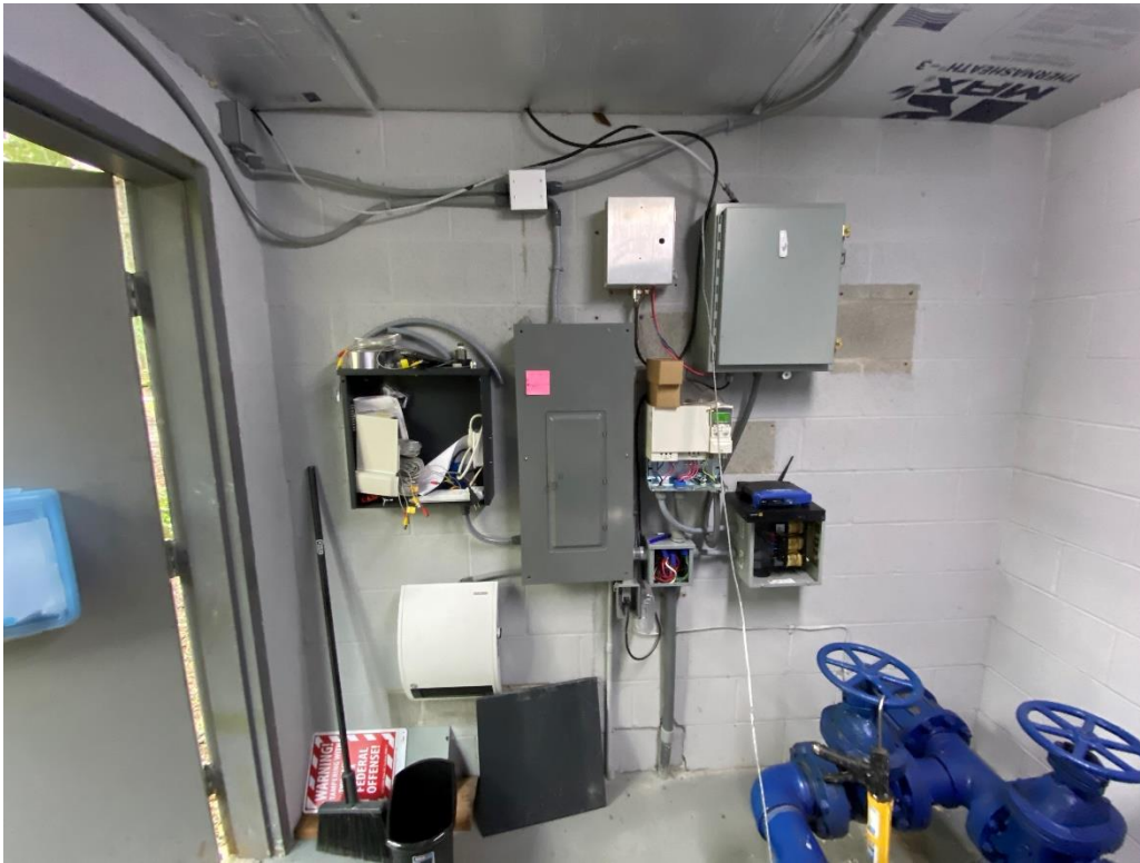
Figure 5: Well 5 Electrical Equipment
