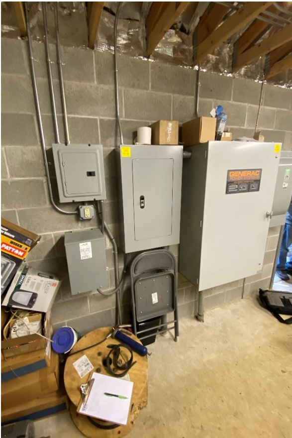
Figure 6: Well 6 Electrical Equipment
