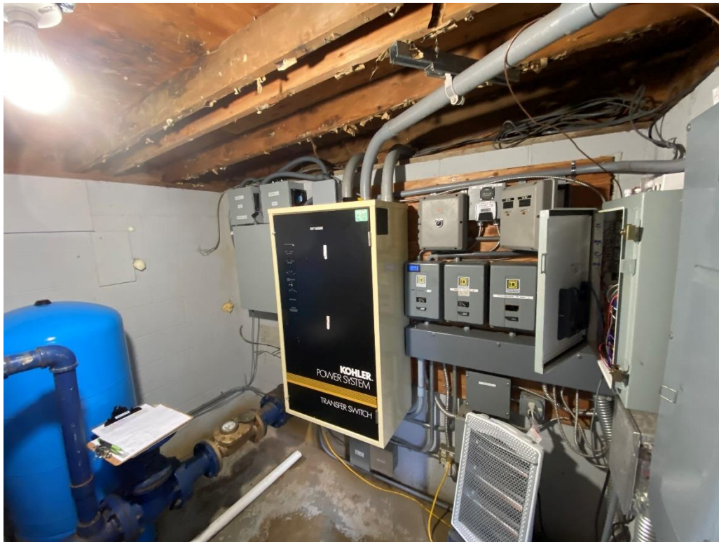
Figure 3: Well 3 Electrical Equipment
