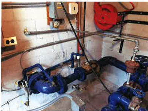
Well House Piping
