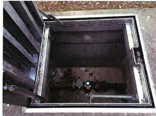
Source Meter Vault
