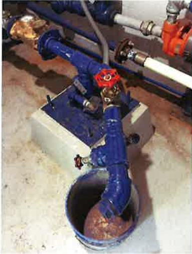
Well #2 – Physically Disconnected
