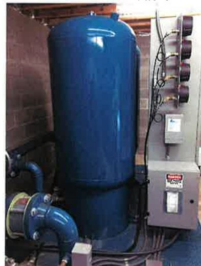
Booster Station Skid
