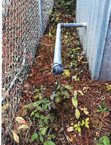
Discharge Line from Booster Station
